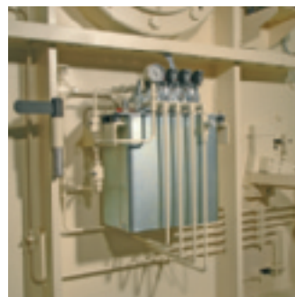
Main hydraulic unit
